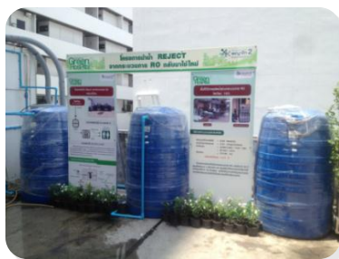
Reuse of rejected water from RO Water.
