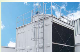
空調裝置 Air-conditioning installation
