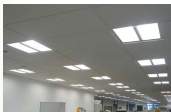
照明裝置 Lighting installation
