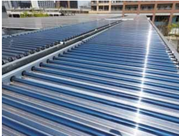
Solar heat panel
