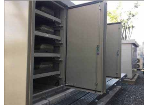
Re-use lithium-ion battery
