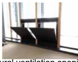
Natural ventilation opening (automatic control)
