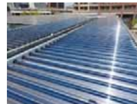
Solar heat collecting panel
